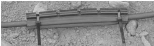
3. Install cable ties at outermost notches of snap lock. Splice is complete.
